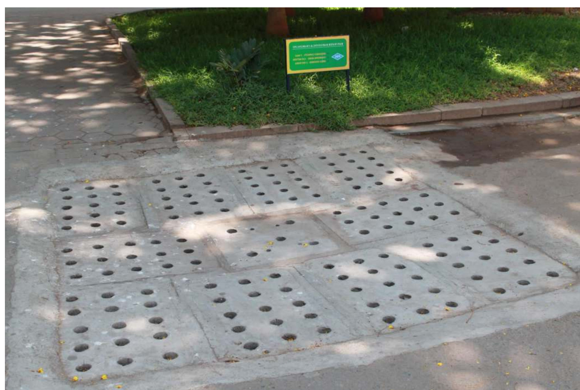
PSG Tech Civil Works - Rain Water Harvesting – Western Side of E Block of Campus
